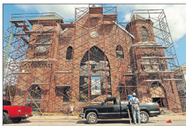
Renovations to the exterior masonry of St. Andrew's Church in 2006. Trying to help save the historic structure was one of the first times DARE expanded its work outside the traditional downtown area. [STARNEWS FILE]
