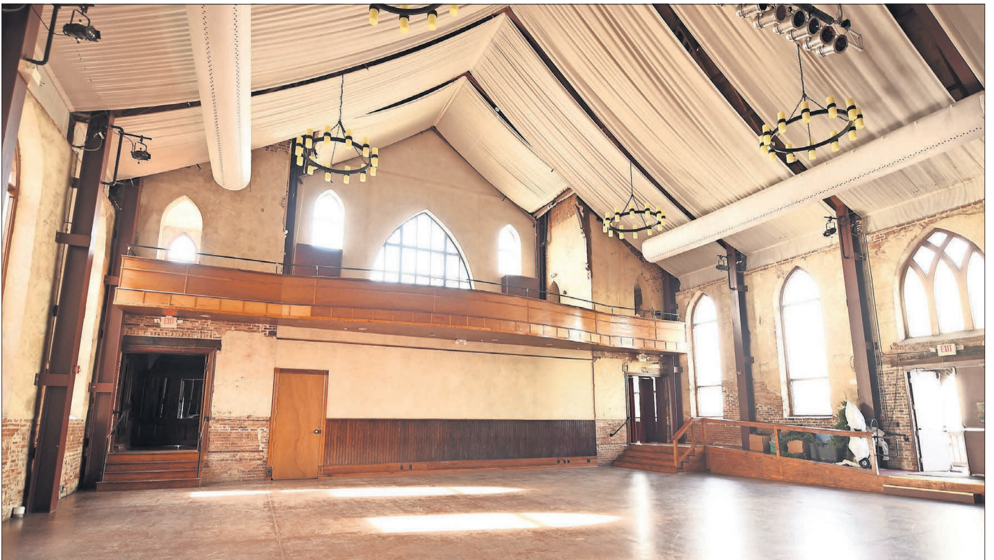
The interior of St. Andrews Presbyterian Church after restoration. The building is now the Brooklyn Arts Center. [STARNEWS FILE PHOTOS]
